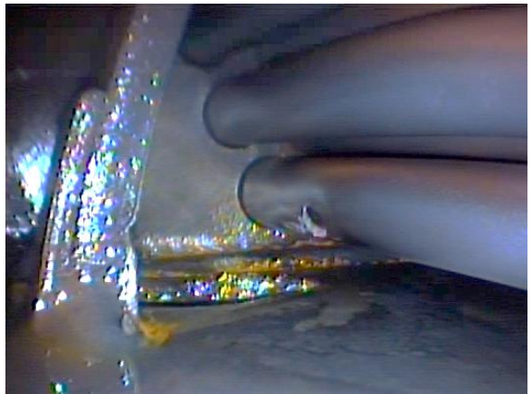
Figure 6 -Shell side video probe of Desuperheating (DSH) Zone inlet window shows damage to bottom plate as well as tube failure.
