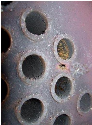
Figure 7 - Tube-to-tubesheet joint weld failure
