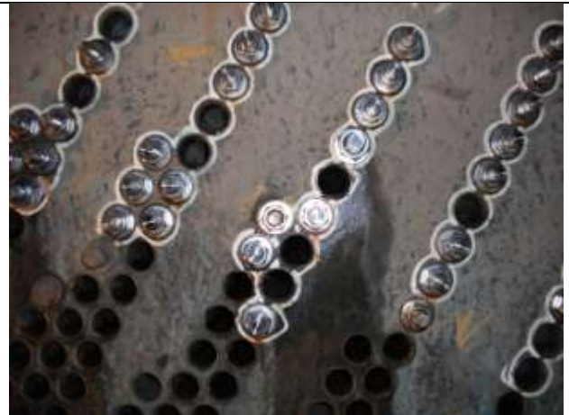
Figure 7 – Condenser tubes following refurbishment. Tubes that passed hydrotest remained unplugged and were returned to service
