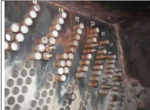
Figure 6 – Condenser Tube plugs prior to testing
